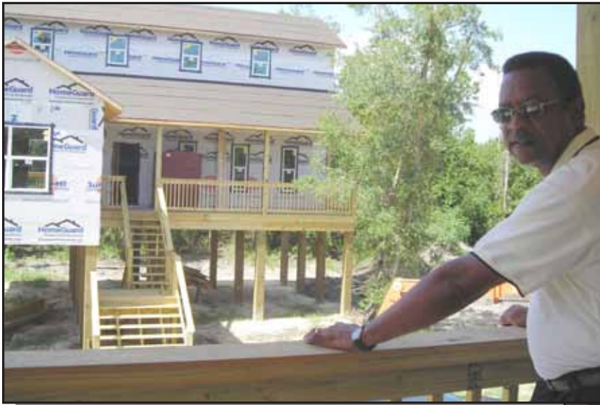
Everett Lewis stands on the porch of Bethel Estates' first model home unit, across the street from the larger, two-story unit that is under construction.
